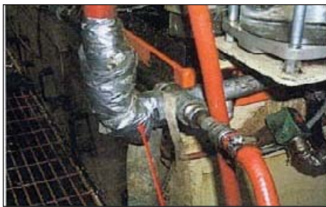
Figure 1A. Some leaks are easy to spot – Look for the duct tape
