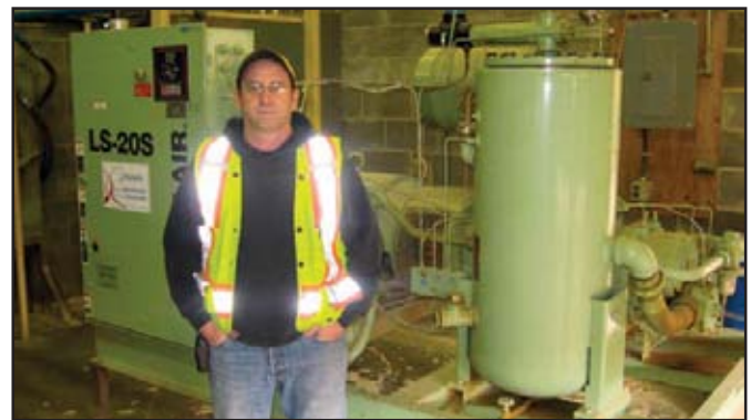
Roger Smith, Newpro Plant Manager, beside air compressor.
