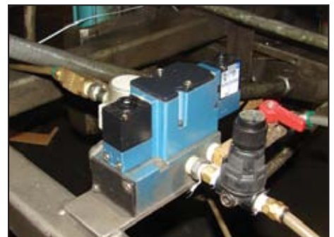
BEFORE: Two 2-position valves consumed 80 cfm when the case packer was idle.
