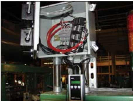
Compressed air flow meters are used on each case erector and flow is displayed and data-logged at a centralized location.
