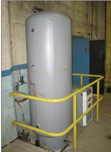
Local storage receivers support pressure caused by intermittent demands.
