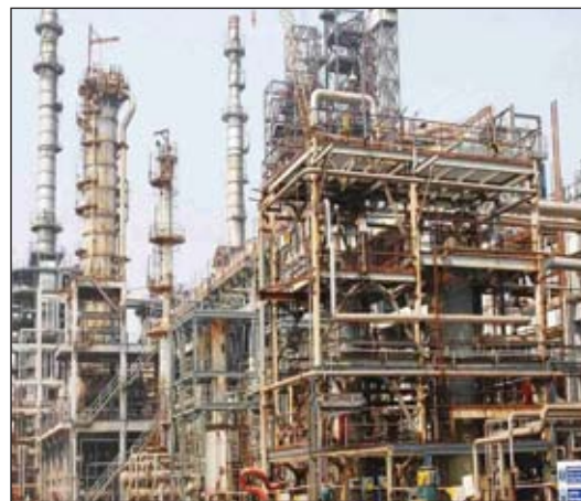
Refineries experience compressed air leaks ranging in severity from Category 1 to Category 3.
