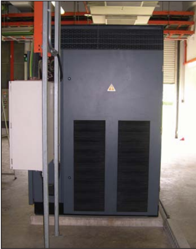
The air compressors were experiencing air intake temperatures above 100 °F. Installing exhaust ventilation duct work on the air compressor helped lower ambient temperatures in the compressor room.
