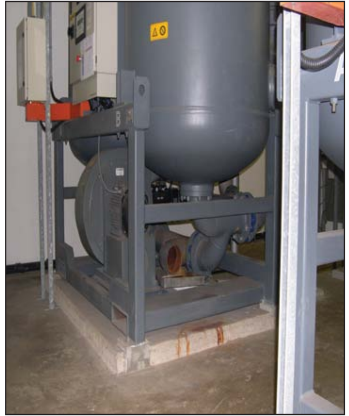
The desiccant air dryer was exhausting 230 °F hot, humid air into the compressor room during the 4-hour regeneration cycle.
