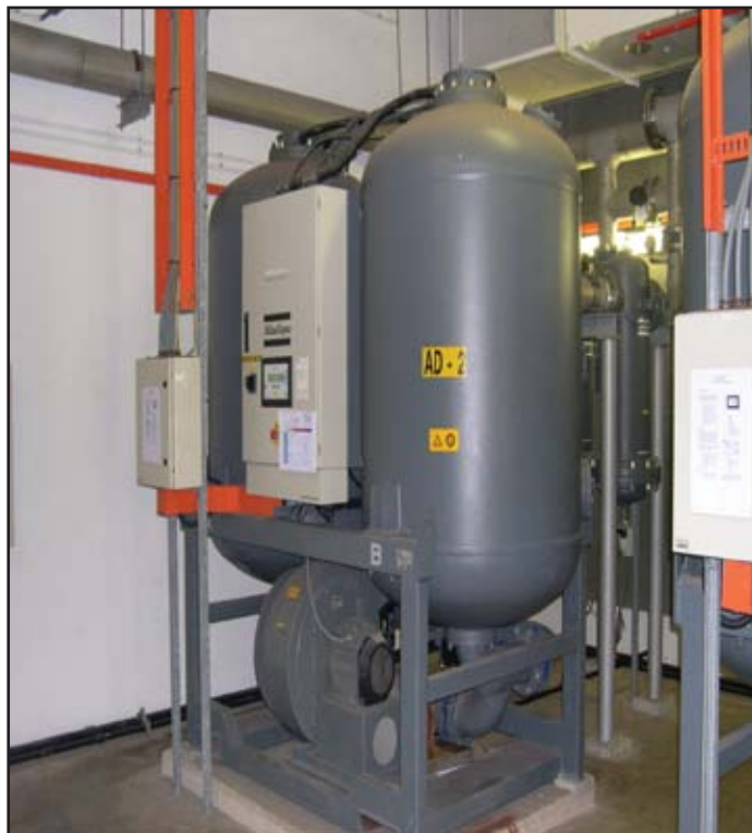
The heated desiccant air dryers, with pre- and after-filters provided a reliable pressure dew point of -40 °F, with a low system pressure drop, for this pharmaceutical plant.
