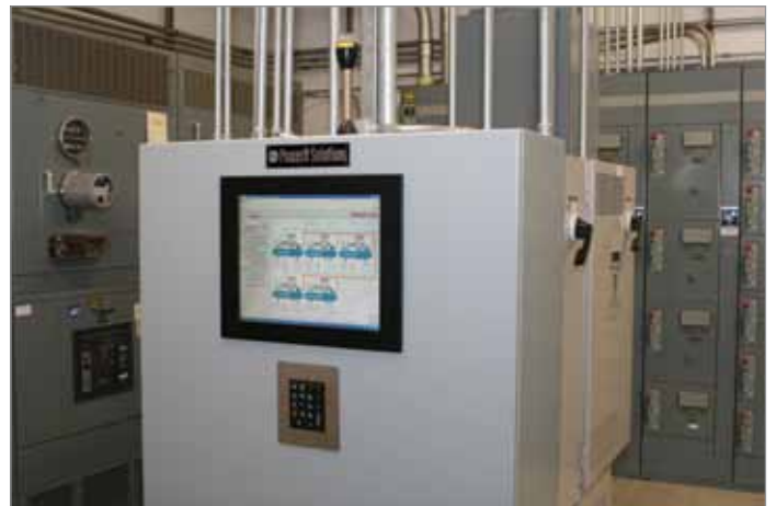
Panel view of the Spara EMS in the main electrical control room at Four Star Fruit
