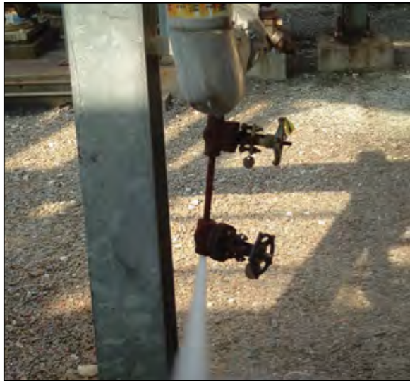
After an ultrasonic test found the trap to be blowing, the downstream condensate line was shut and the test valve was opened to verify test results. The system pressure was 270 psi. At the cost of $10.00 per thousand pounds of steam produced, the energy loss for this single blowing trap is a whopping $21,000.00
