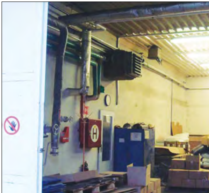
Heater on with door open.
