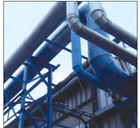
Steam Distribution Piping.
