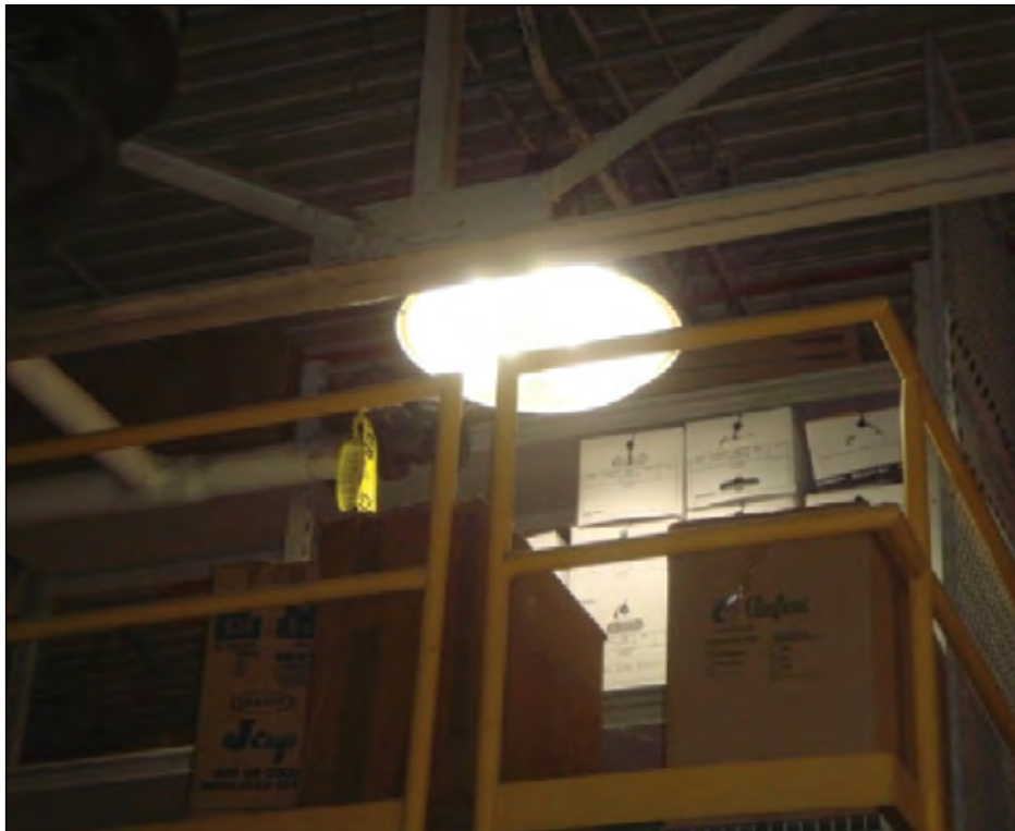
#4 Often light fixtures are obstructed
