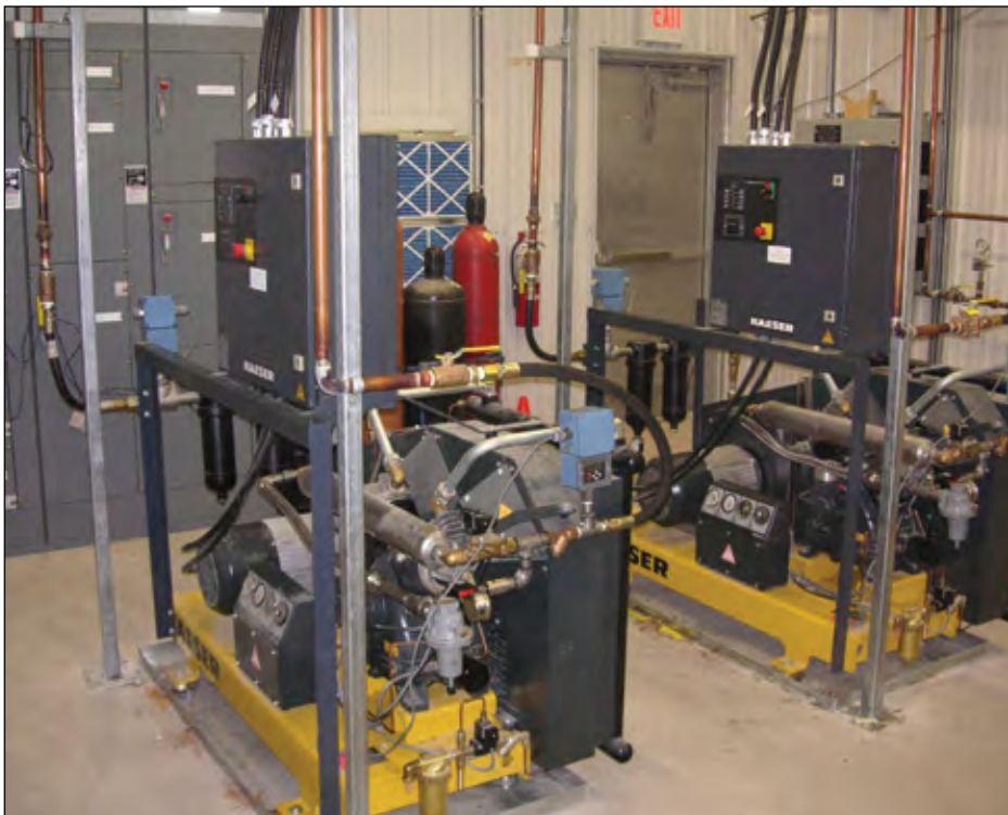
Booster Compressors charge a large 30,000 storage tank to 330 psi
