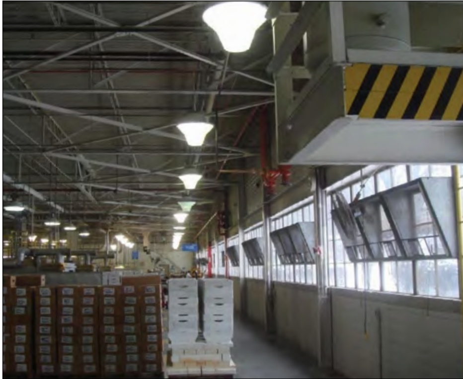
#3 Lights near windows are wasting energy.
