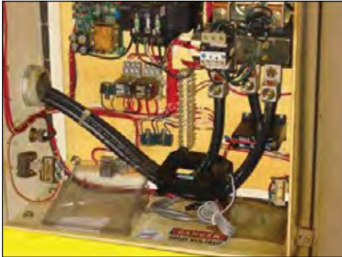
Figure 3: The data logger is installed in the equipment power cabinet
