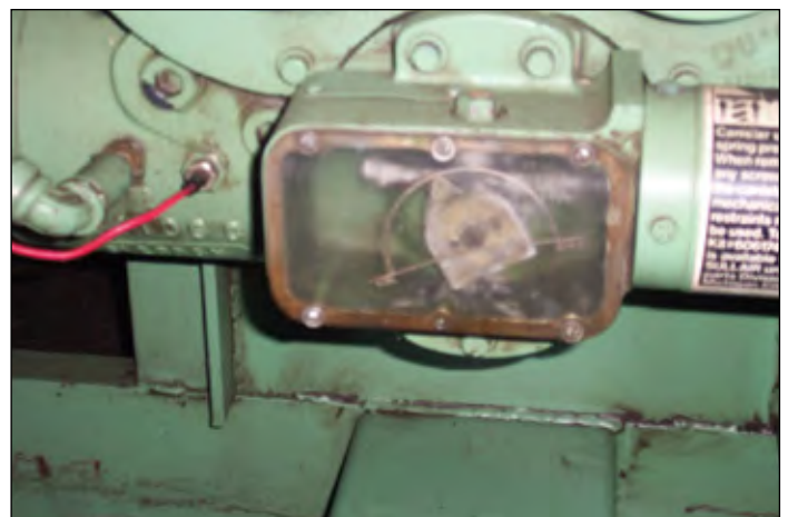
Capacity Controls like this are controlled by a simple screwdriver adjustment. Incorrect adjustment can greatly affect the efficiency of the compressor.
