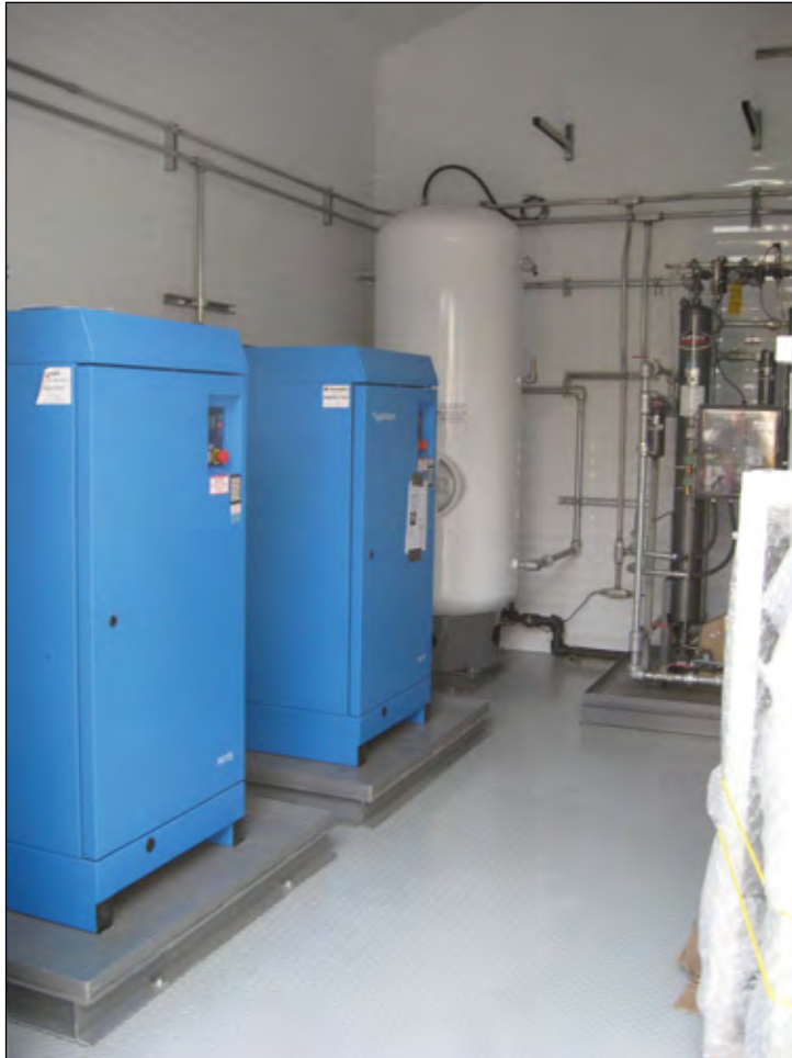
This building contains redundant rotary vane air compressors, a wet air receiver and a regenerative desiccant dryer — all under a PLC controller for remote control.
