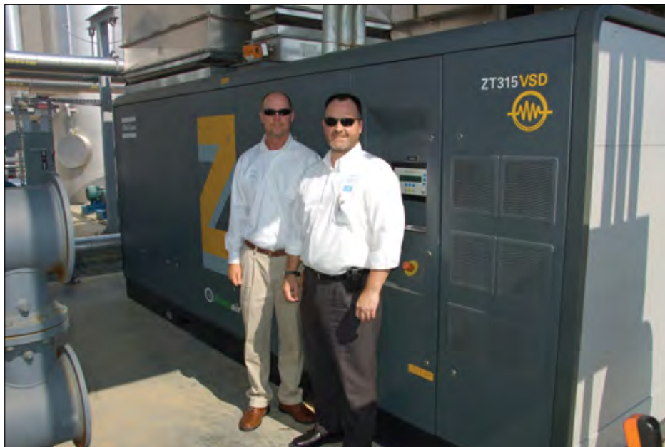
Left to Right: Carl Cline (Haas CNC Racing) and Jim Bruce (Atlas Copco) with the on-site oil-free rotary screw compressors at Windshear Inc.
