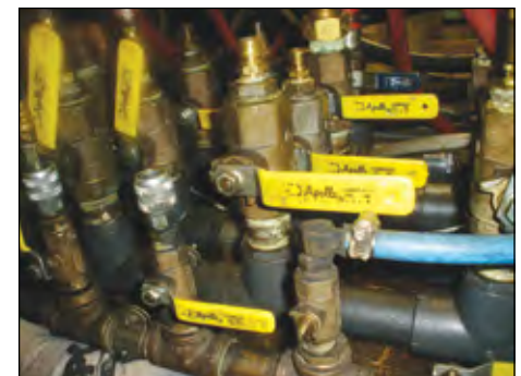
Air leak on hose/fitting connect
