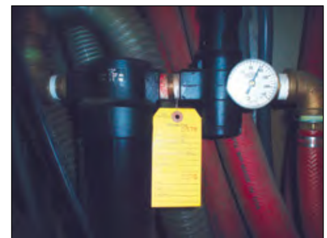
Air leak on FRL
