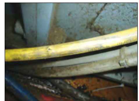
Multiple holes/leaks in tubing
