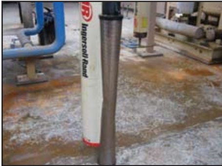
A damaged filter element
