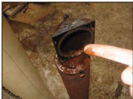
Poor maintenance led to blocked air filters and dryers creating a pressure drop of 35 psig
