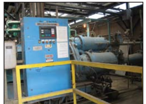
The turn-down controls made this centrifugal oil-free compressor consume 70% of full-load electrical capacity while operating at 40% load — 24 hours per day.
