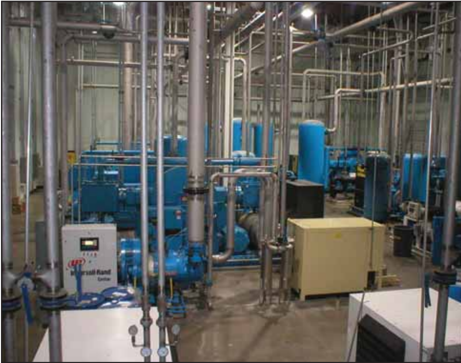
High-Pressure Compressor Room at PET Facility
