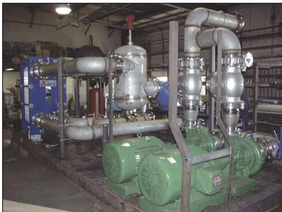
Compressor Cooling System
