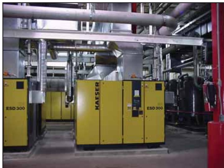
Kaeser Air-Cooled Rotary Screw Compressor at Paper Mill
