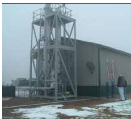
Step 4: Gas Cleaning
