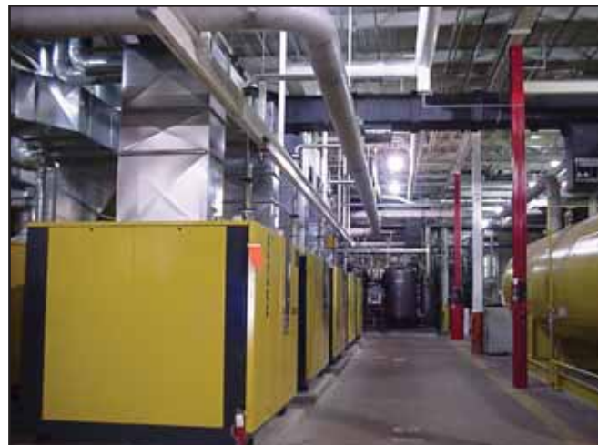
Air-cooled Compressors Provided Water Savings of 1.5 million gallons per day
