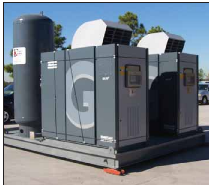
Custom skid package of two 100 horsepower air compressors, a refrigerated dryer, and a receiver tank. Installed at a petrochemical facility along the Houston ship channel.
