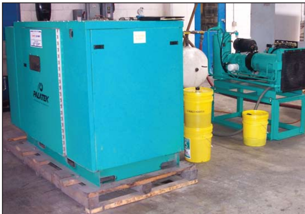
Air compressors installed at a food packaging manufacturer.
