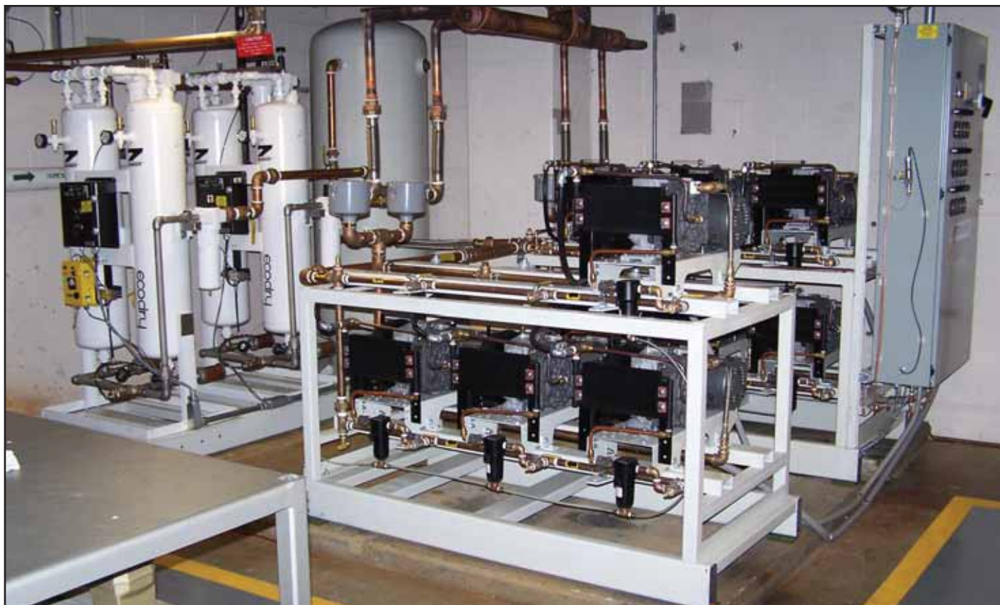
Medical Air Installation With Desiccant Air Dryers
