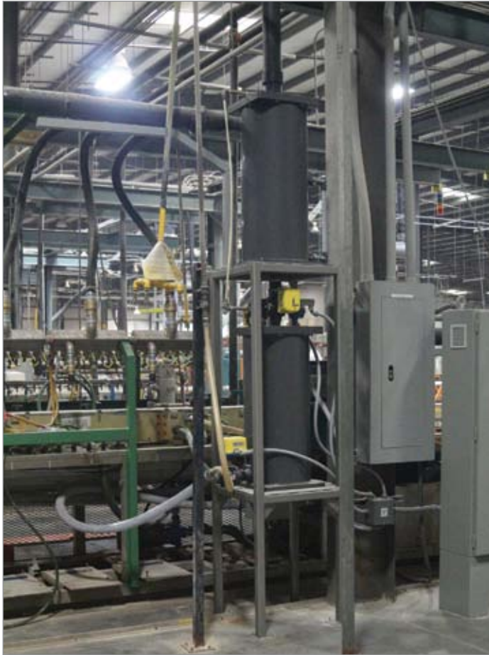
The water separation system for the dry pumps at the calibrator.
