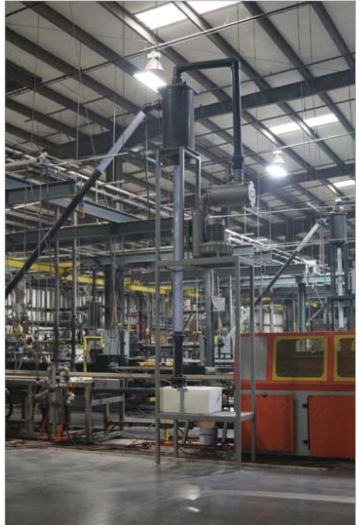
The water separation system for the dry pumps at the tank line.
